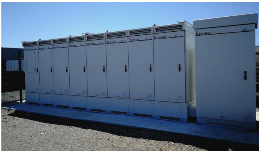
Plate 3-5: Typical centralised inverter (without an enclosure)
