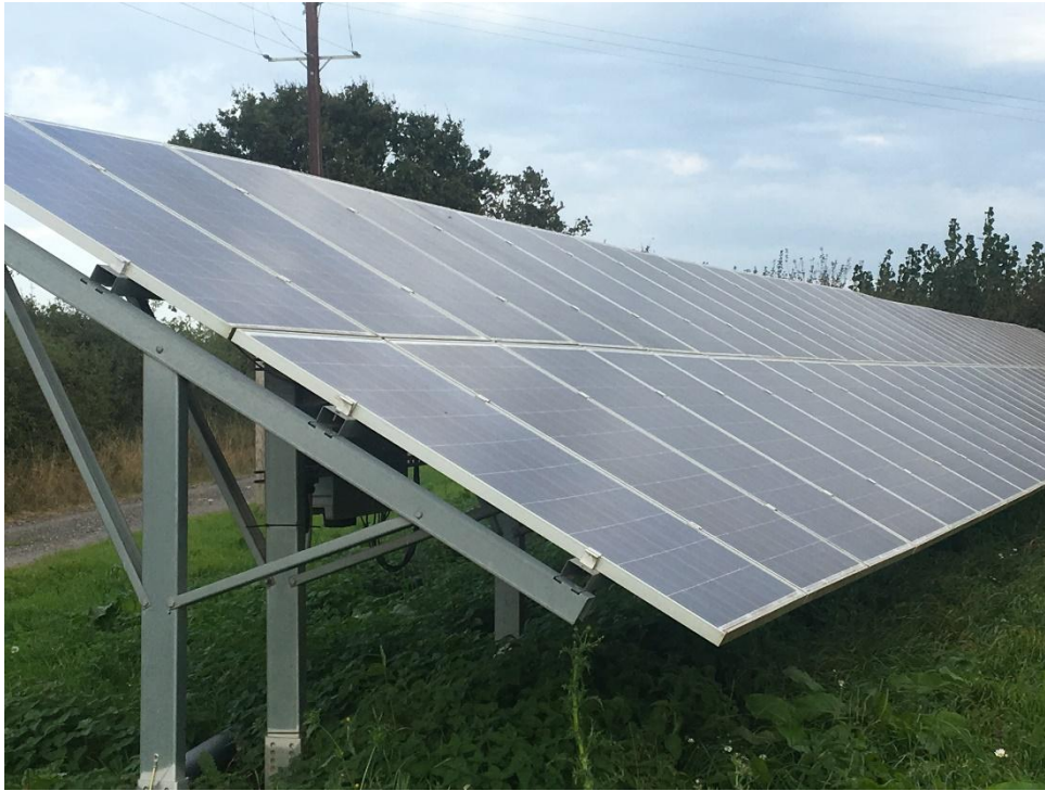
Plate 3-2: Solar panels with south facing configuration
