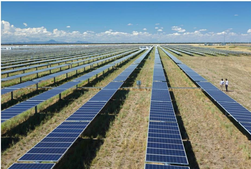
Plate 3-3: Solar panels with single tracker arrays (in the middle of the day)
