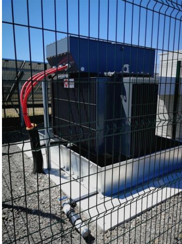
Plate 3-6: Typical transformer (without enclosure)
